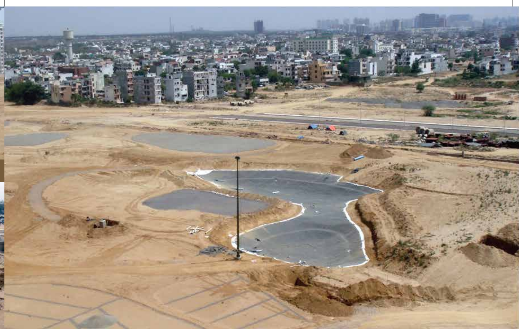
Work in progress – lake lining, capping of tees, greens, light mast erection
